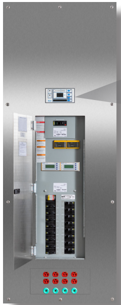
Isolated Power System (IPS)
