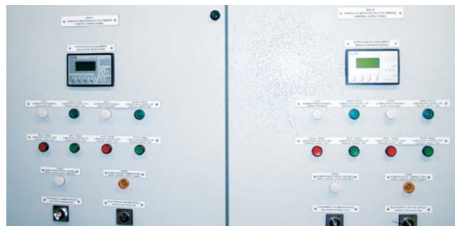
Two of three monitors in operation
