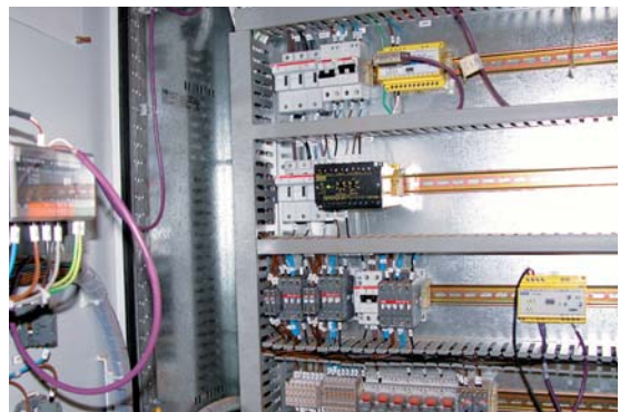
Inside Area 350 switchboard room
