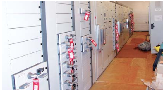
Area 350 switchboard room
