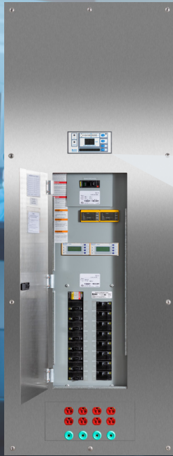
Bender's Isolated Power System (IPS) Panel
